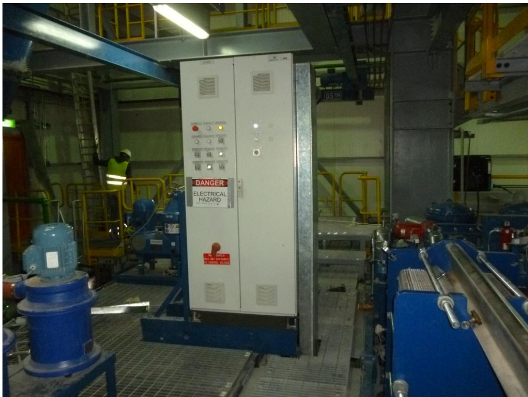
Figure 1. The energized BJA panel, located on top of the pipe module. /21/
