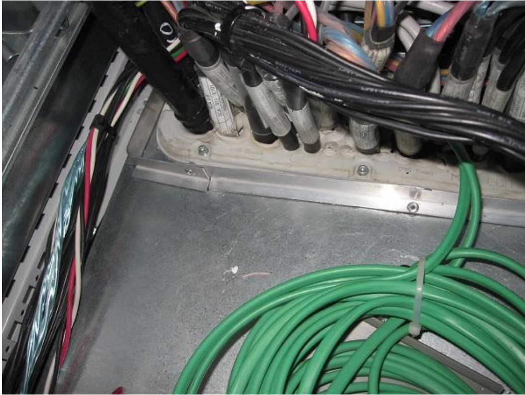
Figure 20. Membrane gaskets that have been done carelessly /21/
