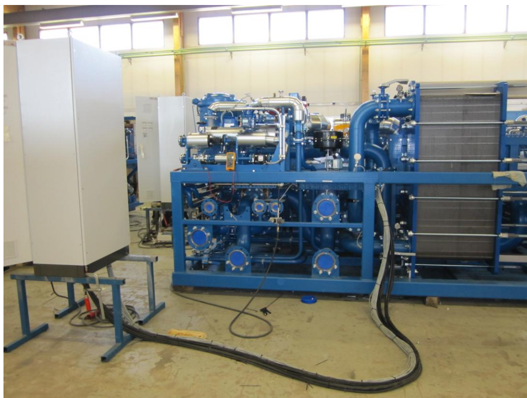
Figure 2. Slack of cables between Engine Auxiliary Module and BJA panel. /21/
