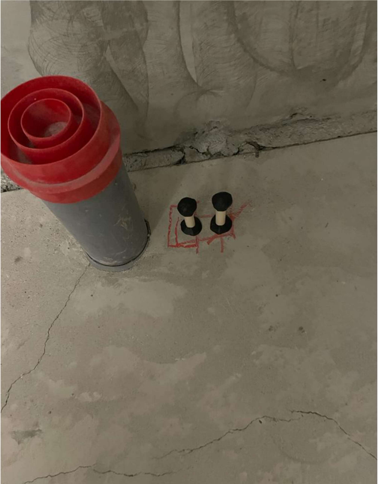
Figure 11 shows a cracked slab
