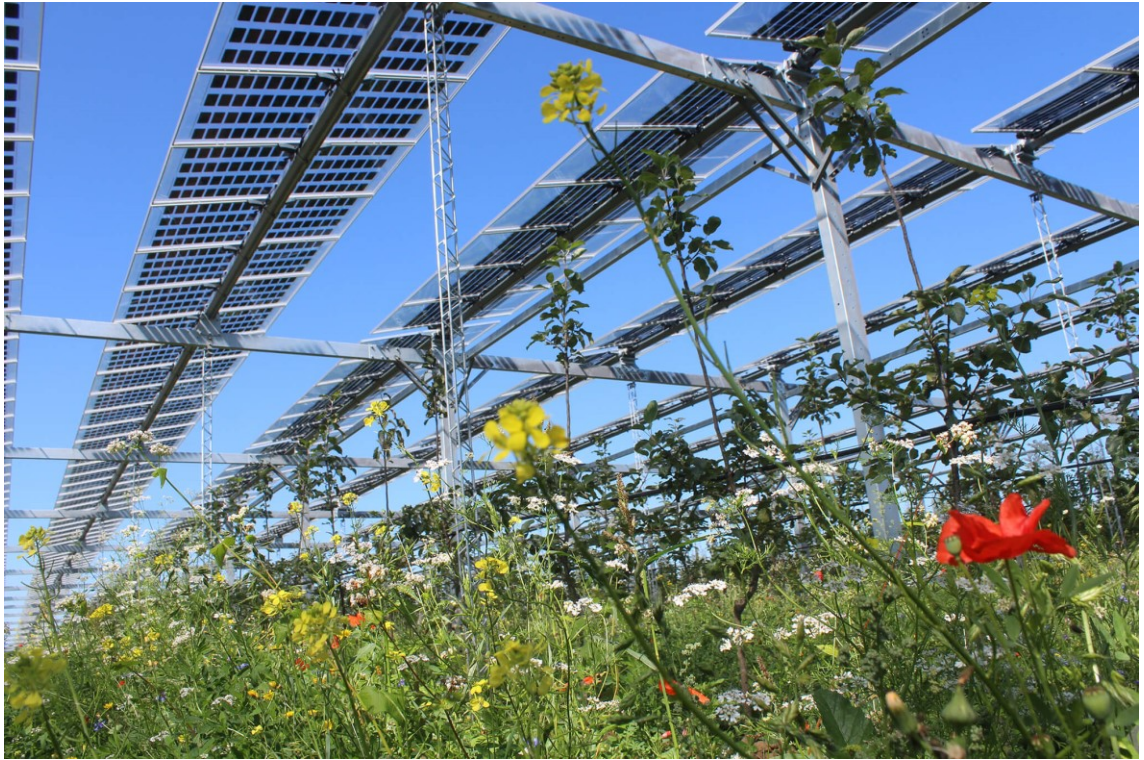
Figure 9. The agrivoltaic site at Gelsdorf, Germany (Fraunhofer ISE 2023).
