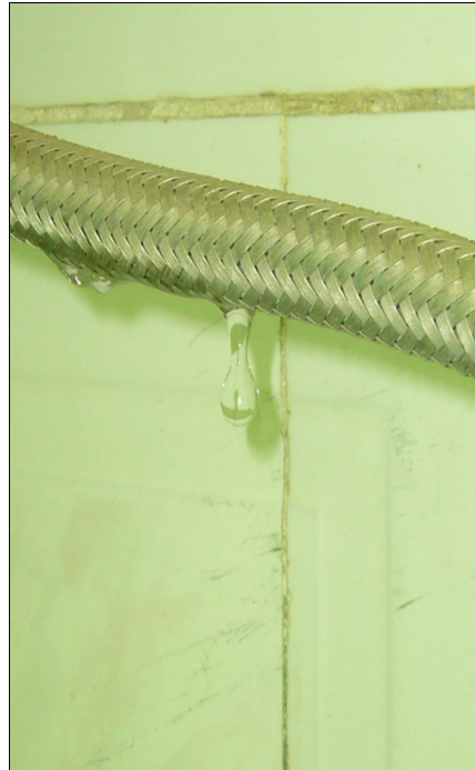
Fig. 8: Leaking water pipe in a hotel bathroom, Bahir Dar 2009 /37/
