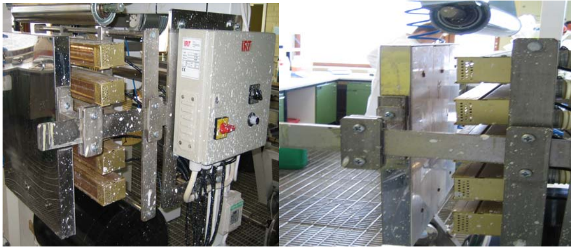
Figure 14 Infrared drying unit and control panel
