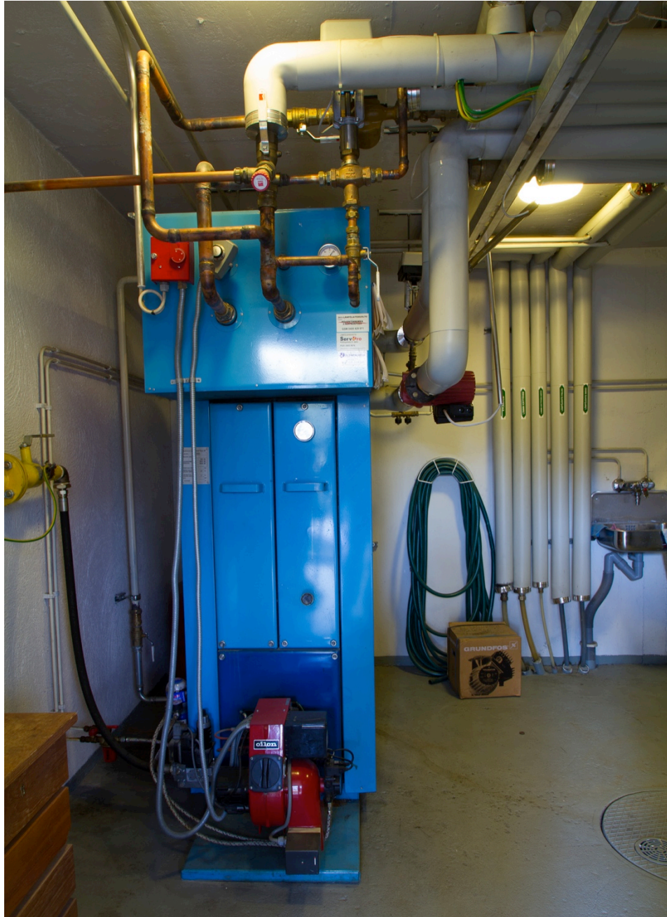
FIGURE 18. Details of the current heating system. Burner, boiler and circulation pump pictured.
