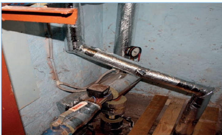
Figure 4. The technical room pipelines, after insulation
