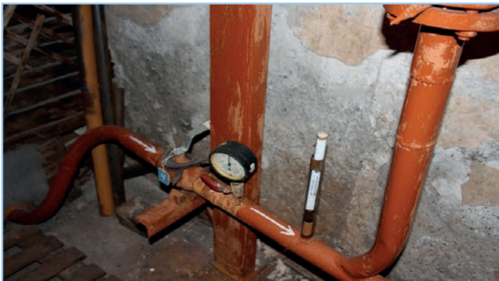
Figure 3. The technical room of the district heating meters and piping before insulation
