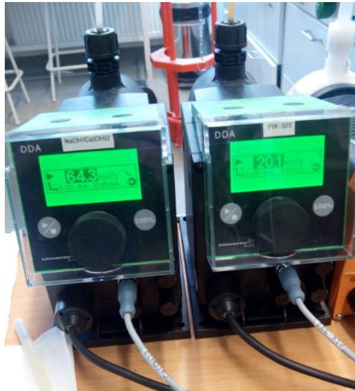
Picture 8. Coagulant and NaOH pump (Miguel Rodríguez del Egado, 2015)
