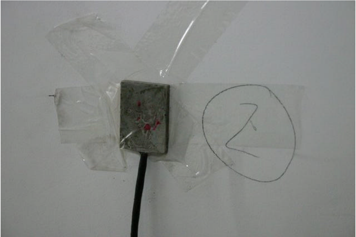
Picture4- 4, Temperature sensor on the wall.
