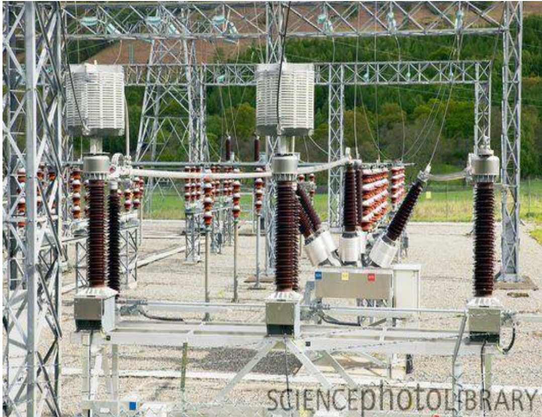
Figure 3. Hydroelectric power substation. /7/
