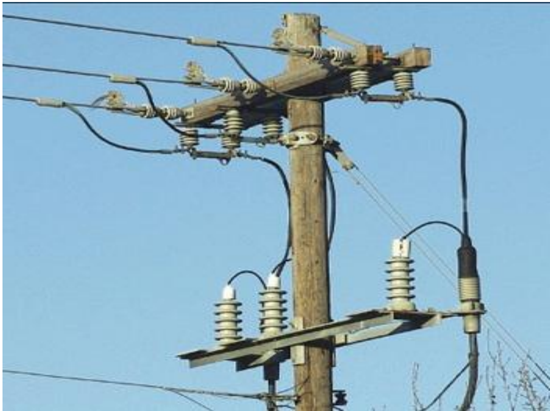
Figure 5. An old pole mounted Disconnector /9/
