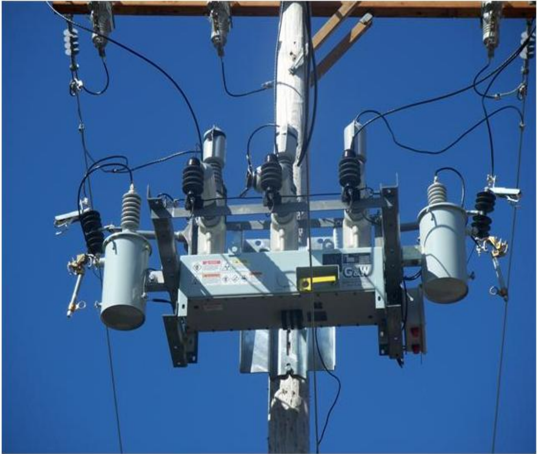
Figure 4. Pole mounted Recloser /8/
