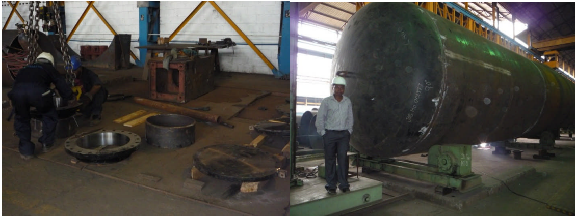
PICTURE 4 & 5. Construction progress of manhole and pressure vessel for Chevron by the C.E.O. (Photos: Femi Adefolalu 2007)
