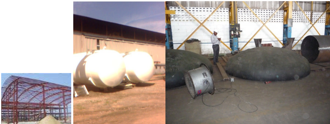
PICTURE 1, 2 & 3. Structural steel works for Mercedes Benz warehouse, ground tanks for Shell Nigeria Ltd and Pressure Vessel Dish for Chevron on inspection; executed by the C.E.O (Photos: Femi Adefolalu 2007)
