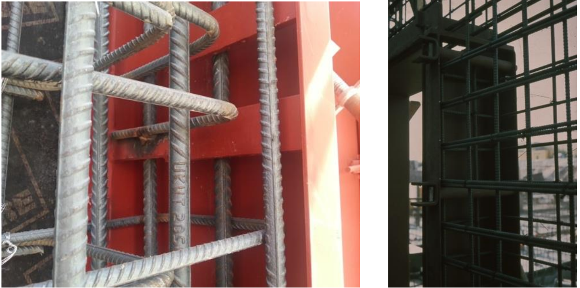
Figure 5 Examples of connection details of the Blast Doors to the concrete wall surround
