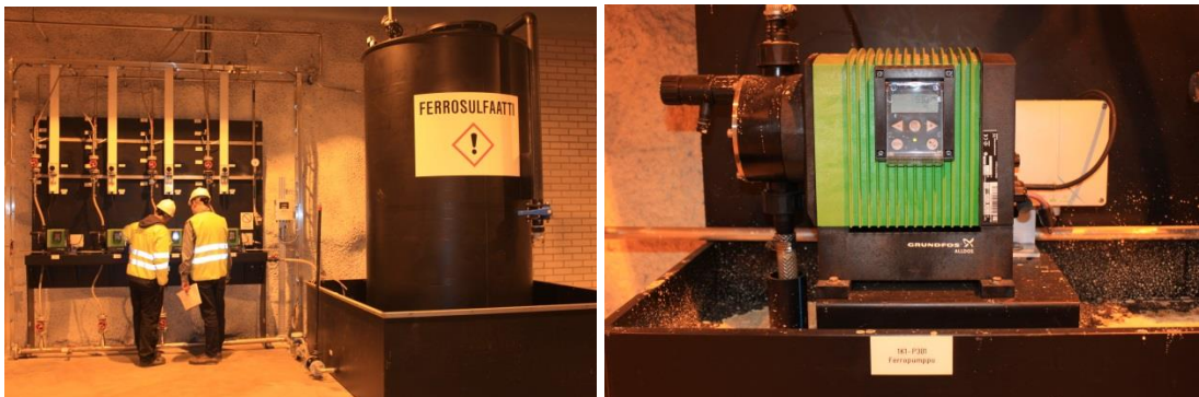
PICTURE 23. dosing skid system with the chemical tank containing iron sulfate. (Photo taken during a customer visit).
