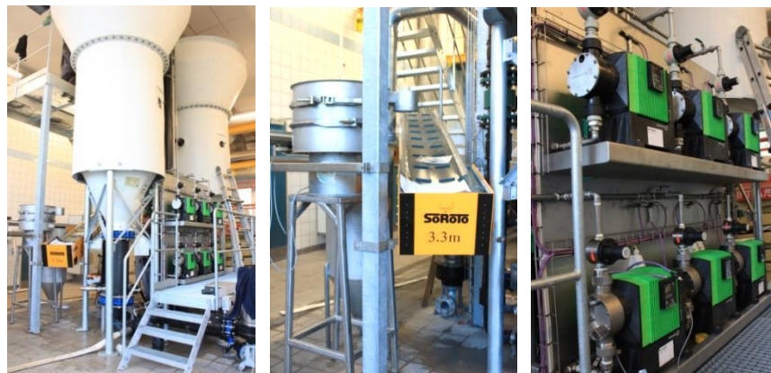
PICTURE 8. Struvite plant and dosing pumps. Photo taken during a customer visit.
