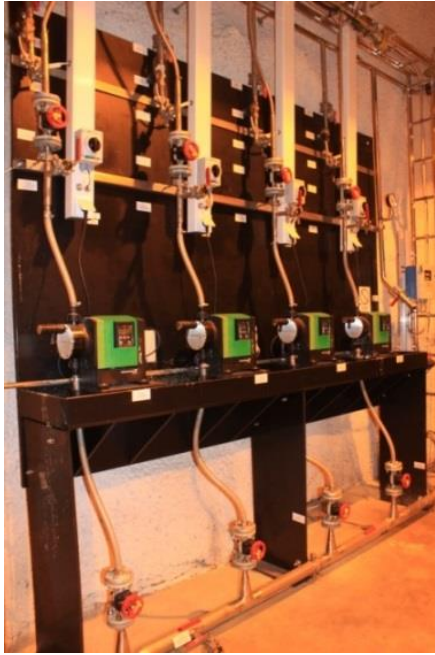
PICTURE 22. Dosing skid/system in Turku WWTP. (Photo taken during a customer visit).
