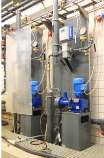
PICTURE 4. Dosing units to be renewed in Lynette WWTP, Copenhagen. Photo taken during a customer visit.
