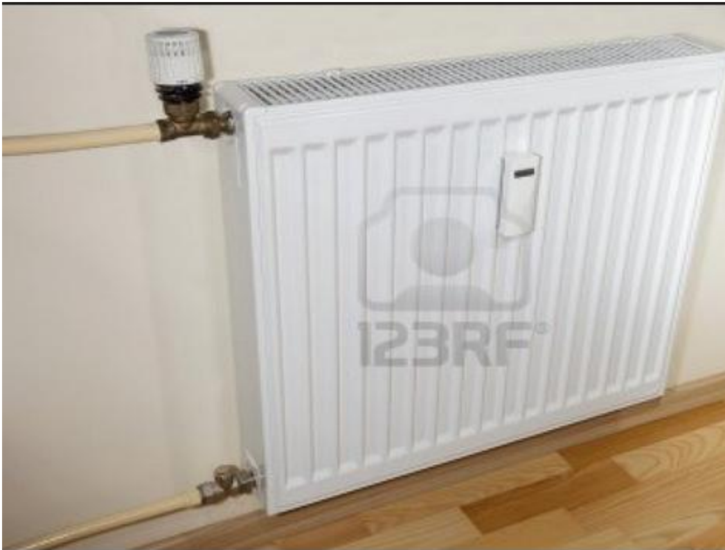
Figure17: The radiator in a room.
