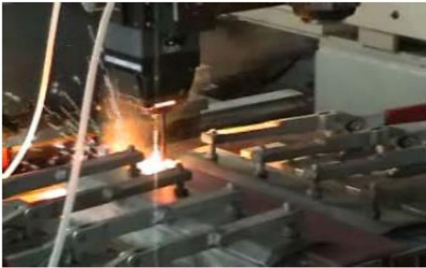
First welding tests with 10.4kW in steel using protective gas and cross jet
