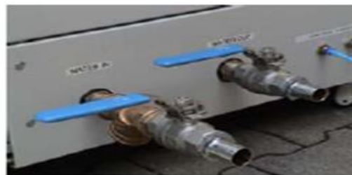
Water supply for the 10kW High Power Fiber Laser
