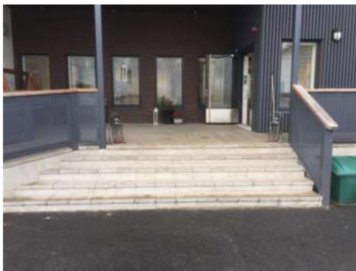
Figure 10: Stairs leading to the front door of the entrance of Villa Toukola
