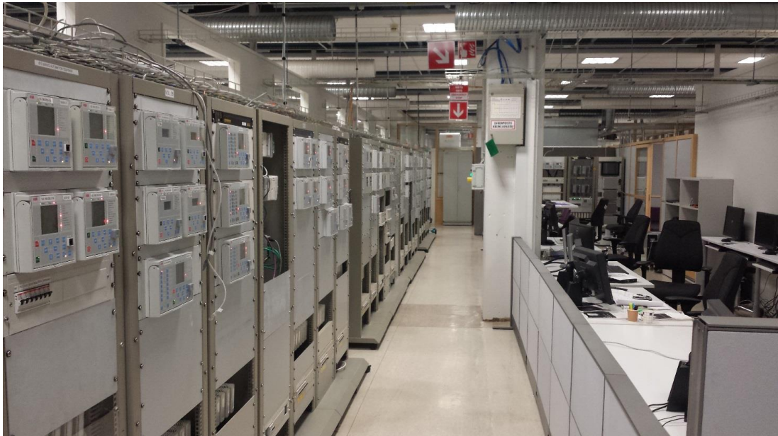
Figure 2. PVC laboratory, ABB Vaasa Finland
