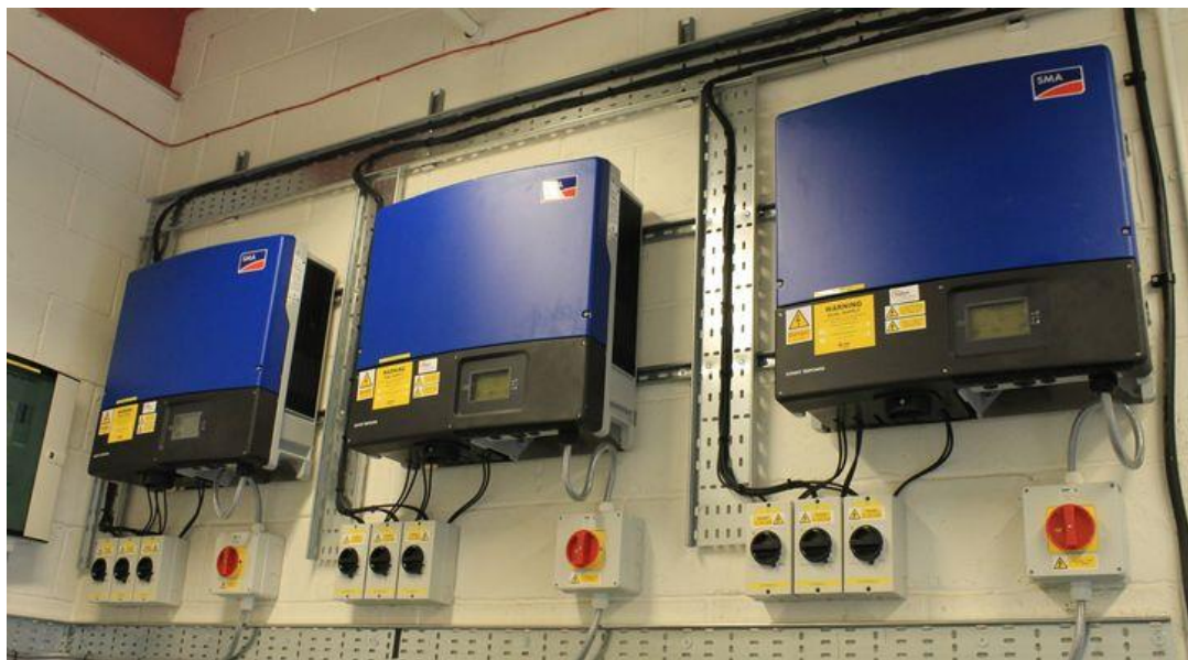
Figure 9. Inverter. (© 2016 Rudge Energy 2016.04.08.)
