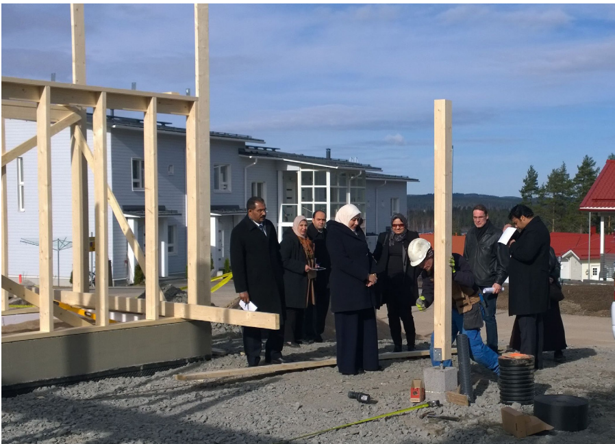
Study visit group getting to know a construction site built by the students of Jyväskylä College
