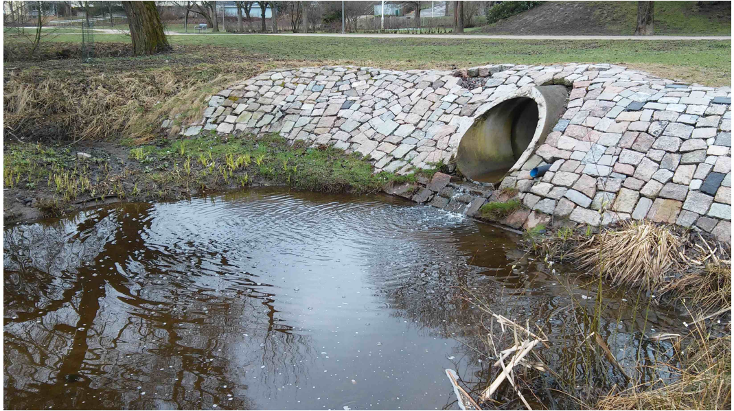
FIGURE 11. The discharge pipe of the urban runoff system of Southern Haaga
