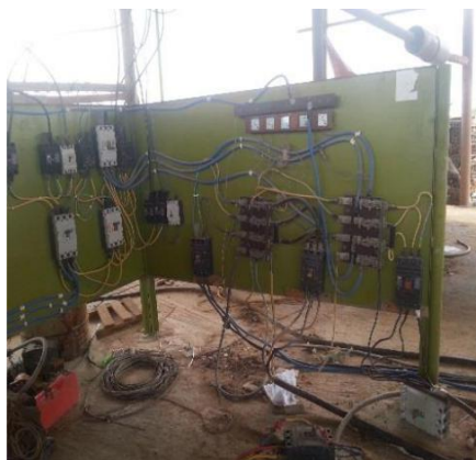
Figure 8 Bus bar arrangement in Adado Electrical Company[20]
