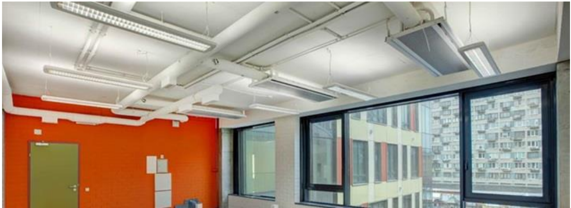
Figure 12. Ventilation system of ECO Status building
