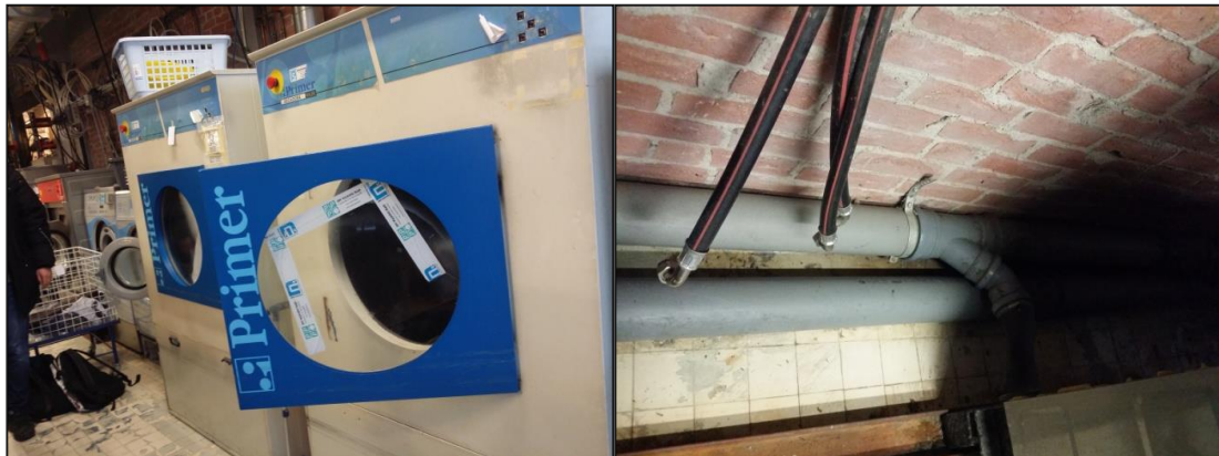
Figure 2. Washing machine and dryer's (a) and washing machine water exit (b)
