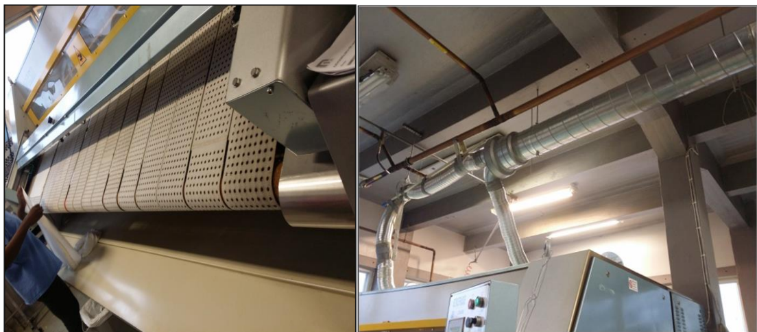
Figure 3. Mangle dryer (a) and dryer exhaust (b)
