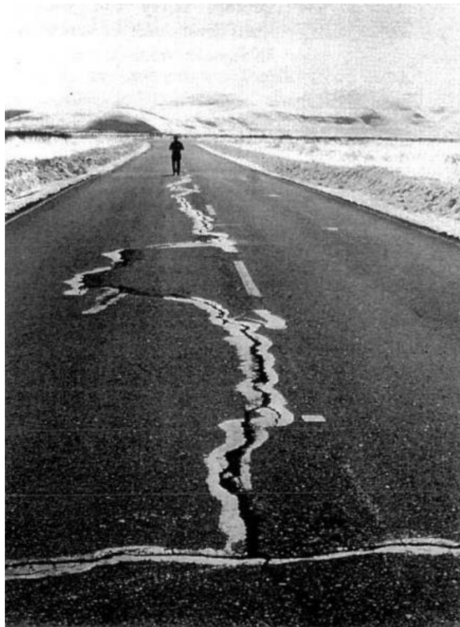
Figure 9. Example of Longitudinal and Transverse Cracking due to Snow Insulated Embankments (Critical Depth of Snow Surpassed) (Rooney & Vinson 1996, 6)
