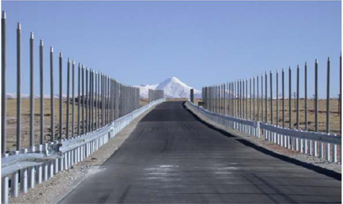
Figure 15. Thermosyphons in China to Maintain the Frozen Condition Below a Roadway Embankment (Shur 2015d)
