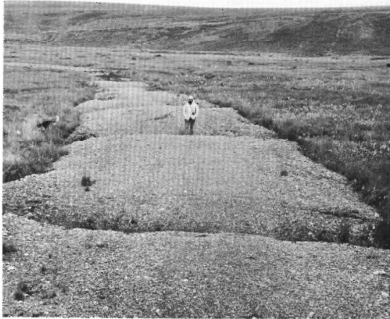
Figure 7. Severe Differential Subsidence on an Abandoned Gravel Road (Ferrians Kachadoorian & Greene, 1969)
