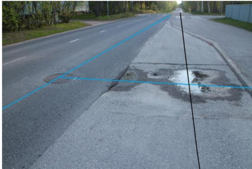
Figure 12. Roadway Faulting by a Bus Stop (Rytlahti 2016)
