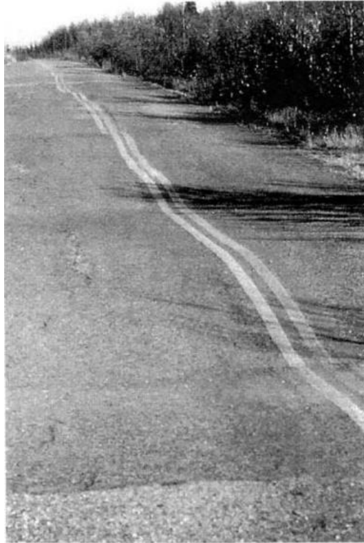
Figure 10. Surface Deformation due to Seasonal Frost Heaving and Permafrost Thawing (Rooney & Vinson 1996, 7)
