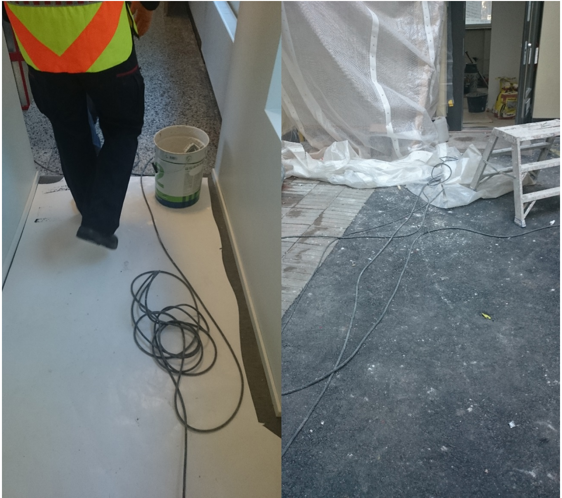
Photograph 2: Cable wires laying around everywhere
