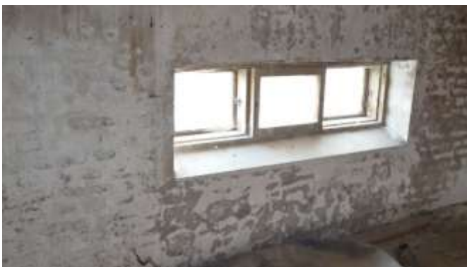
Picture 9: The windows require thorough repair.
