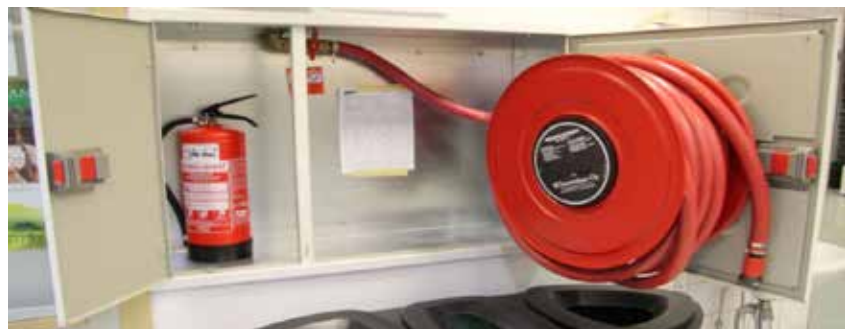
Picture 4. Fire hydrant content
