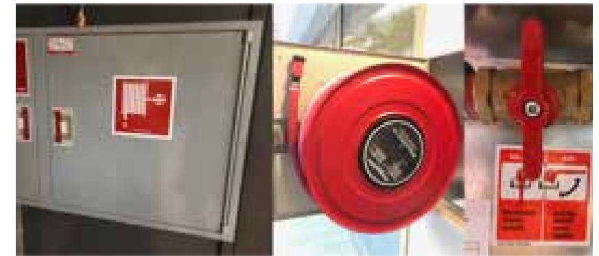
Picture 3. Use instructions of fire hose box
