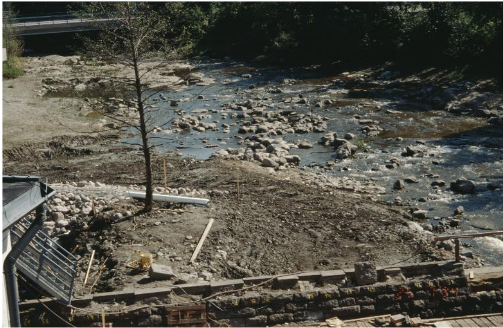
Photo 11. A picture taken from Vernissa towards Kuninkaalantie bridge in 1994 when the technical fish ladder was under construction. The bed rock and numerous stones are visible in the channel. (Keski-Uudenmaan vesiensuojelun liikelaitoskuntayhtymä 1994.)
