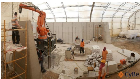
Picture 6. Mobile concrete printer developed by CyBe. The R & Drone laboratory construction field in Dubai which is 3D printed and featured in an article: 3dprint.com, CyBe Construction Announces That 3D Printing is Complete for Dubai's R & Drone Laboratory 2017.
