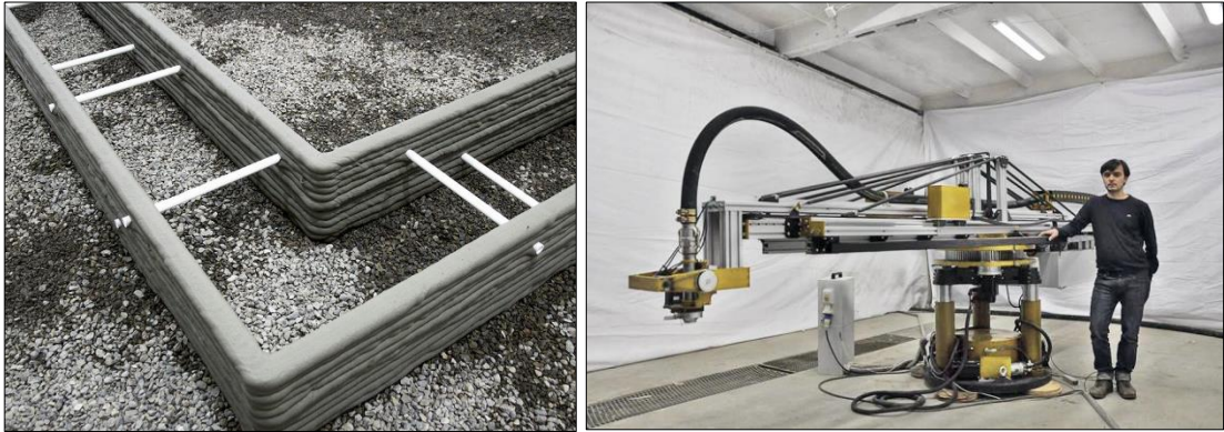
Picture 11. (a) Framework for a building foundation by ApisCor printer. (b) Nikita Chenyun-tai ApisCor inventor and ApisCor printer. Images by ApisCor
