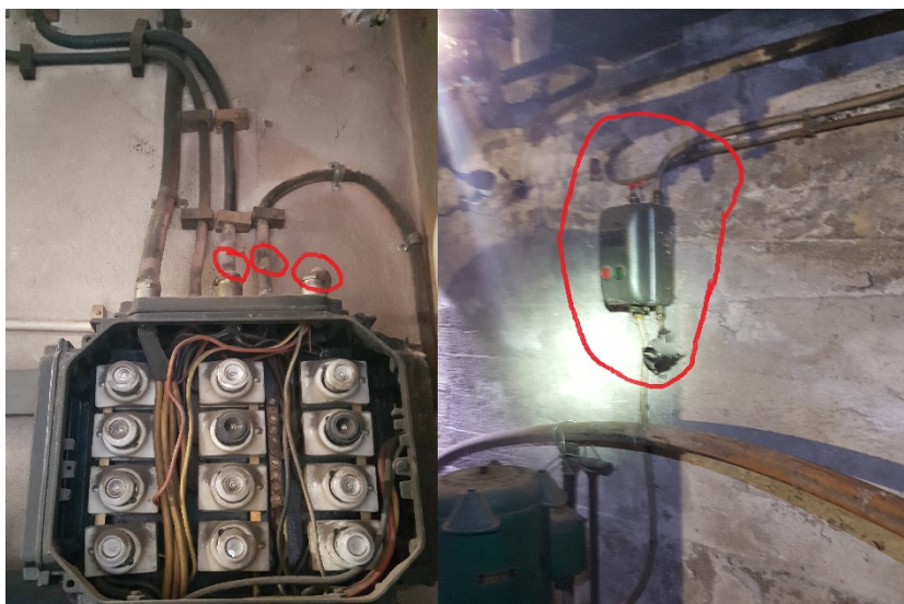
Figure 27 room C Cabinet PK3 & 28 room B system in basement.
