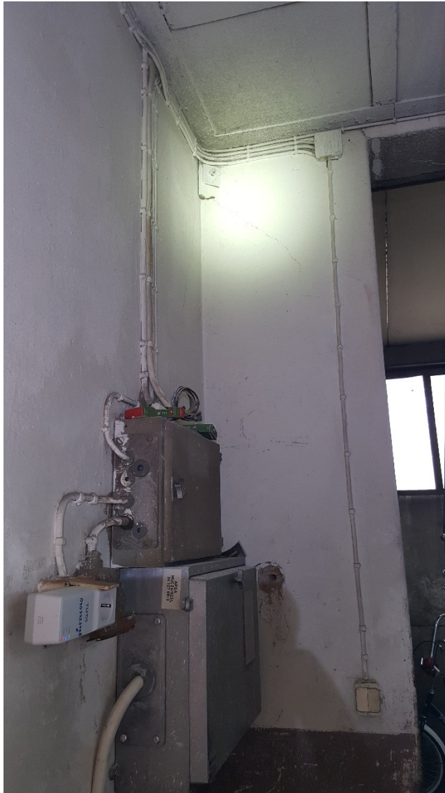
Figure 16 D. Service hall cabinet
