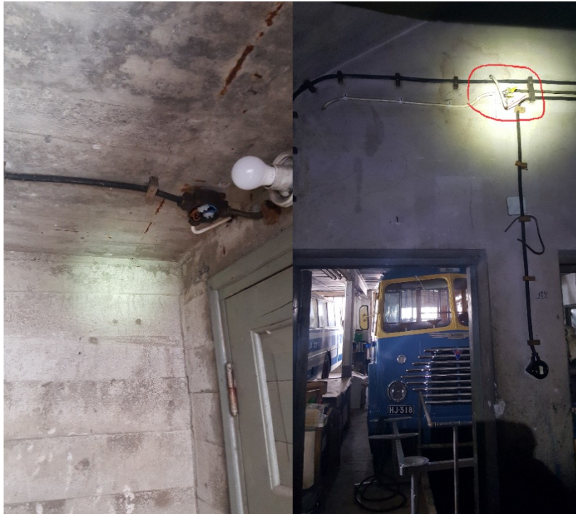
Figure 21 room A Missing cover & 22 room C missing distribution box.
