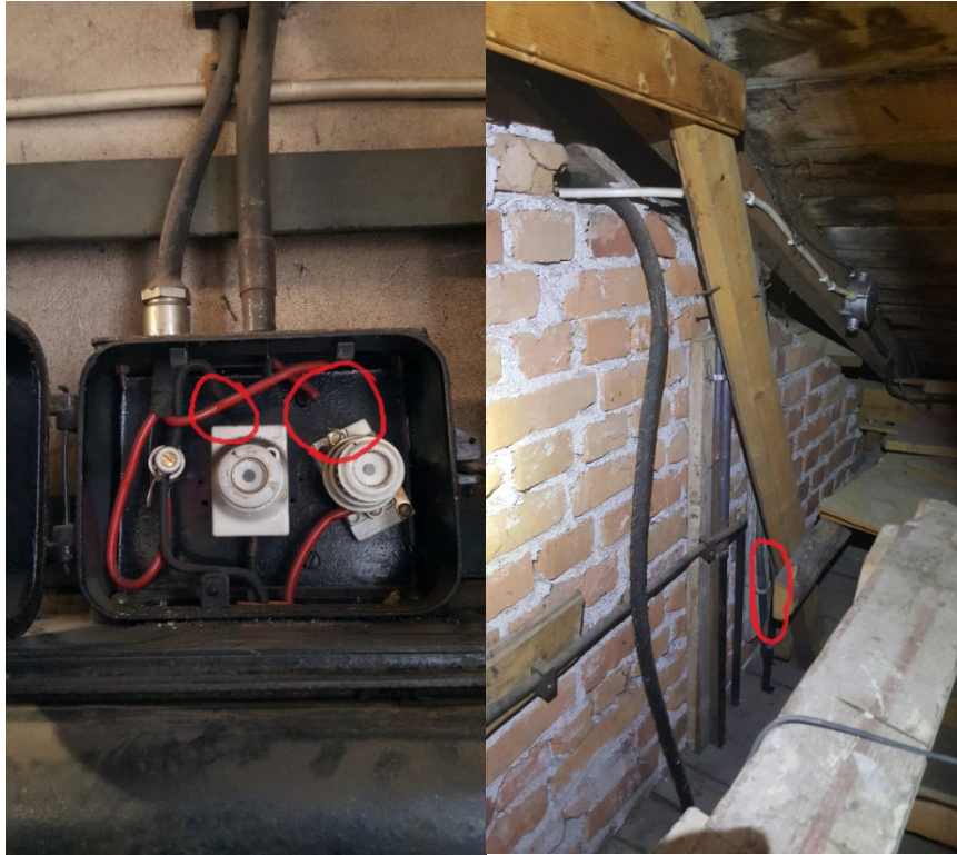
Figure 25 room C Cabinet PK2 & 26 room H corresponding cables on the attic.
