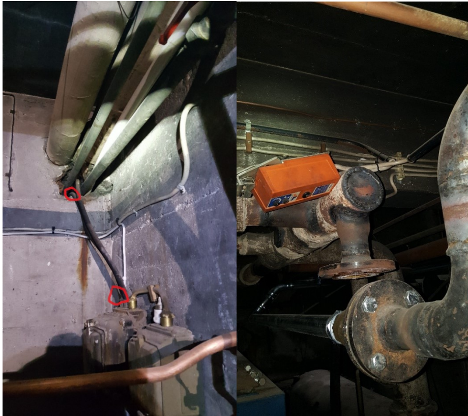
Figures 39 room B Cabinet TT1 old output &40 room B old heating system out of use.
