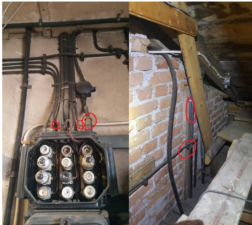
Figure 23 room C Cabinet PK1 & 24 room H cables on the attic.
