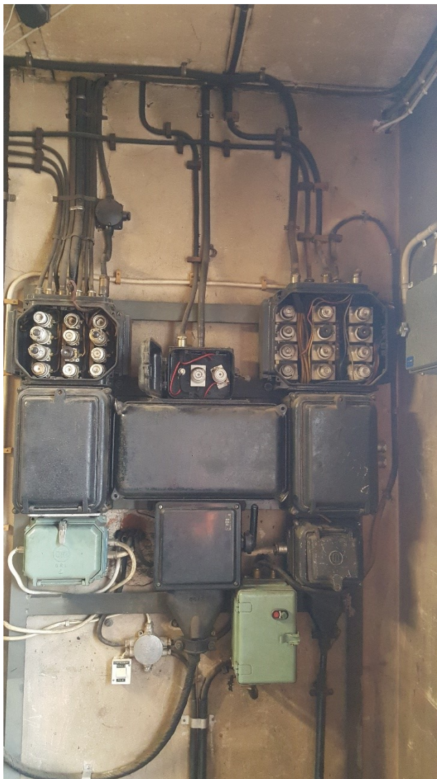
Figure 15 C. Main distribution cabinets.
