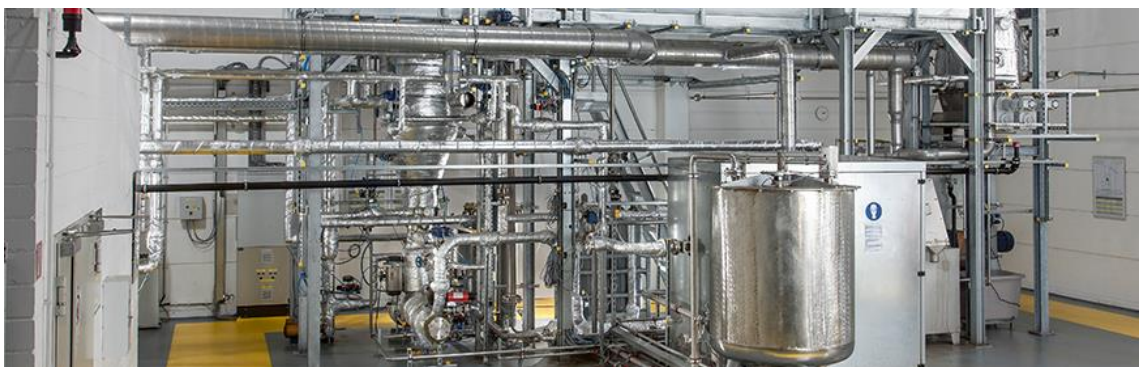
PICTURE 9. HTC pilot plant (Valmet. 2017.)
