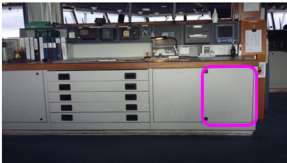
FOG IS LOCATED IN THE CABINET UNDER THE CHART BOARD
