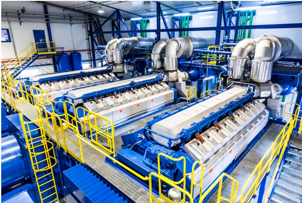
Figure 30. A power plant equipped with Wärtsilä 34SG gas engines. /29/
