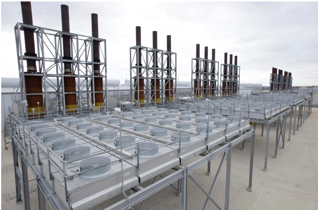
Figure 32. Power plant radiator field. /31/
