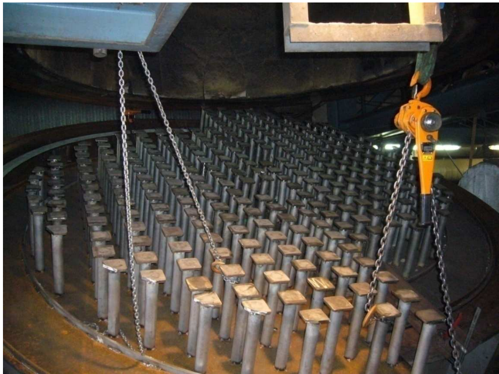
FIGURE 11: The second grate half nearly in position. A gasket tape circling the wind chest is partly visible
