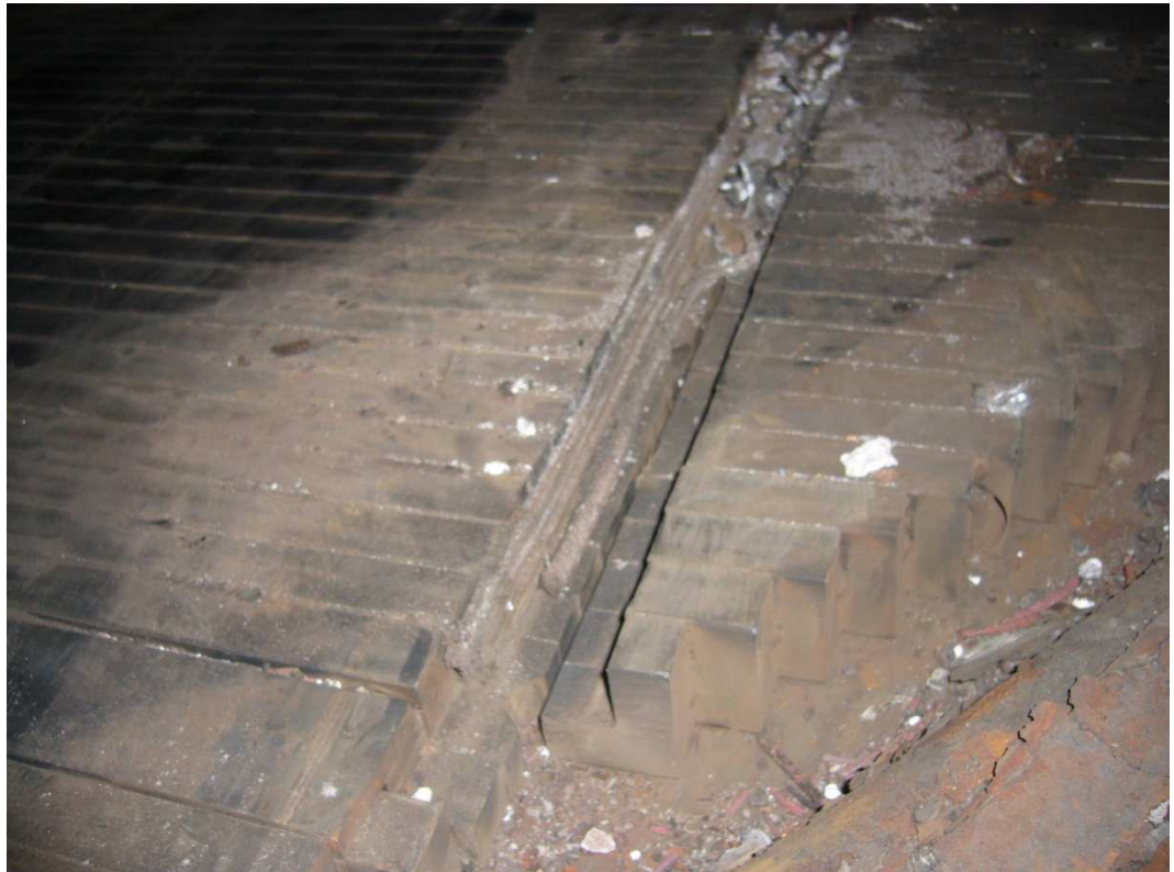
FIGURE 4: Closer examination of the stationary fire grate bars of the KPA boiler prior to retrofitting
