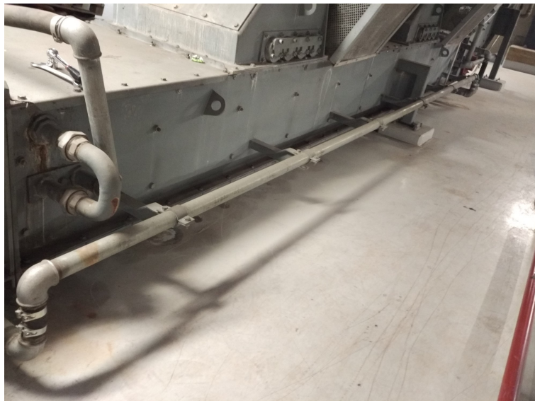
Figure 3: Targeted piping section altered in the experiment
