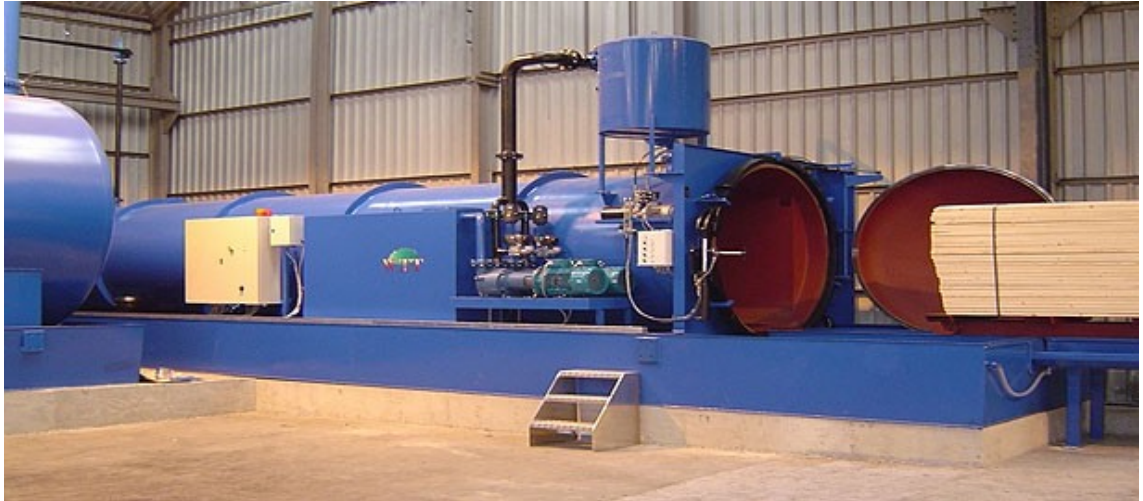
Picture 2. An autoclave at timber impregnation plant (Source: Стандарт Вуд 2018b).
