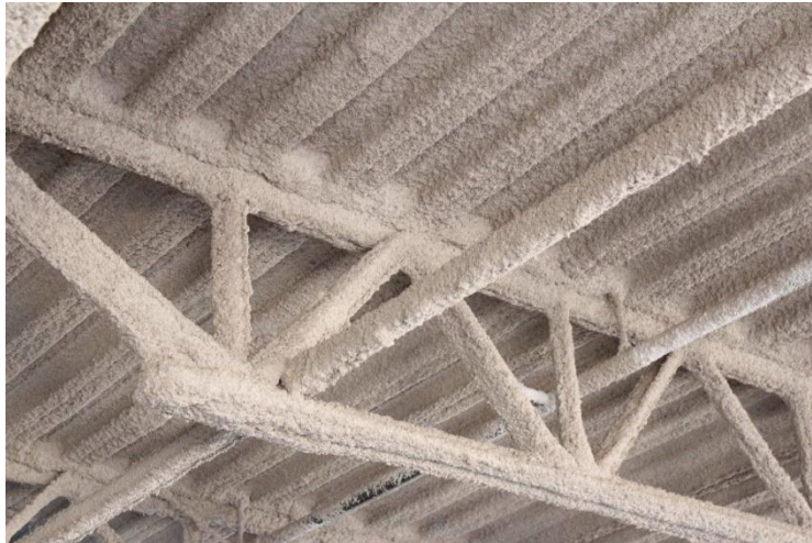
Figure 8. Spray fire protection (4)
