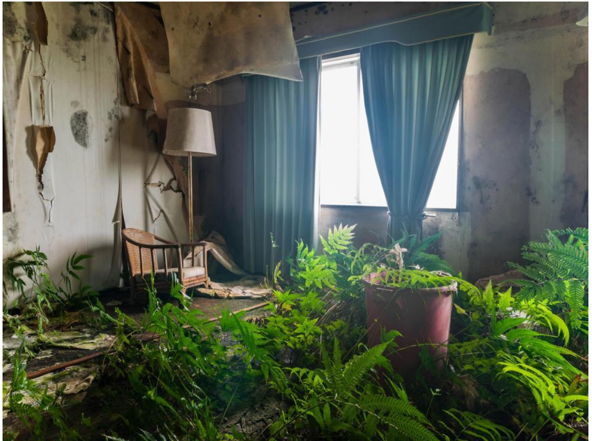
Figure 1. Abandoned hotel room, photograph by Mirebs. The photo shows a room that has fallen into obvious disrepair, likely untouched for a longer period of time.
