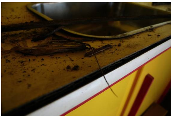
Figure 115. Loose edging strip.
