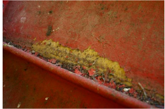
Figure 103. Red paint layer is coming off and gel-coat is exposed.
