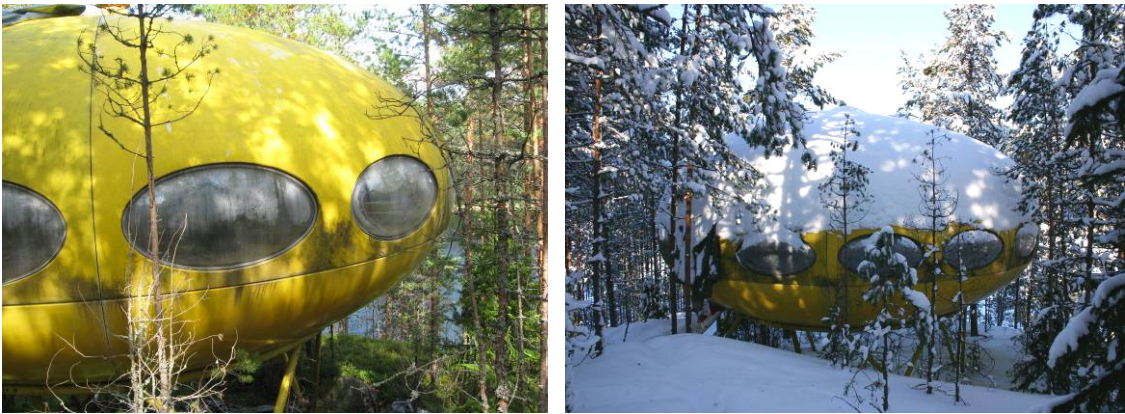
Figure 100. (left) A photograph taken in September 2009 shows the roof condition. Figure 101. (right) Snow covers the roof.
