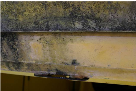
Figure 98. Some cracks are visible above the door.
