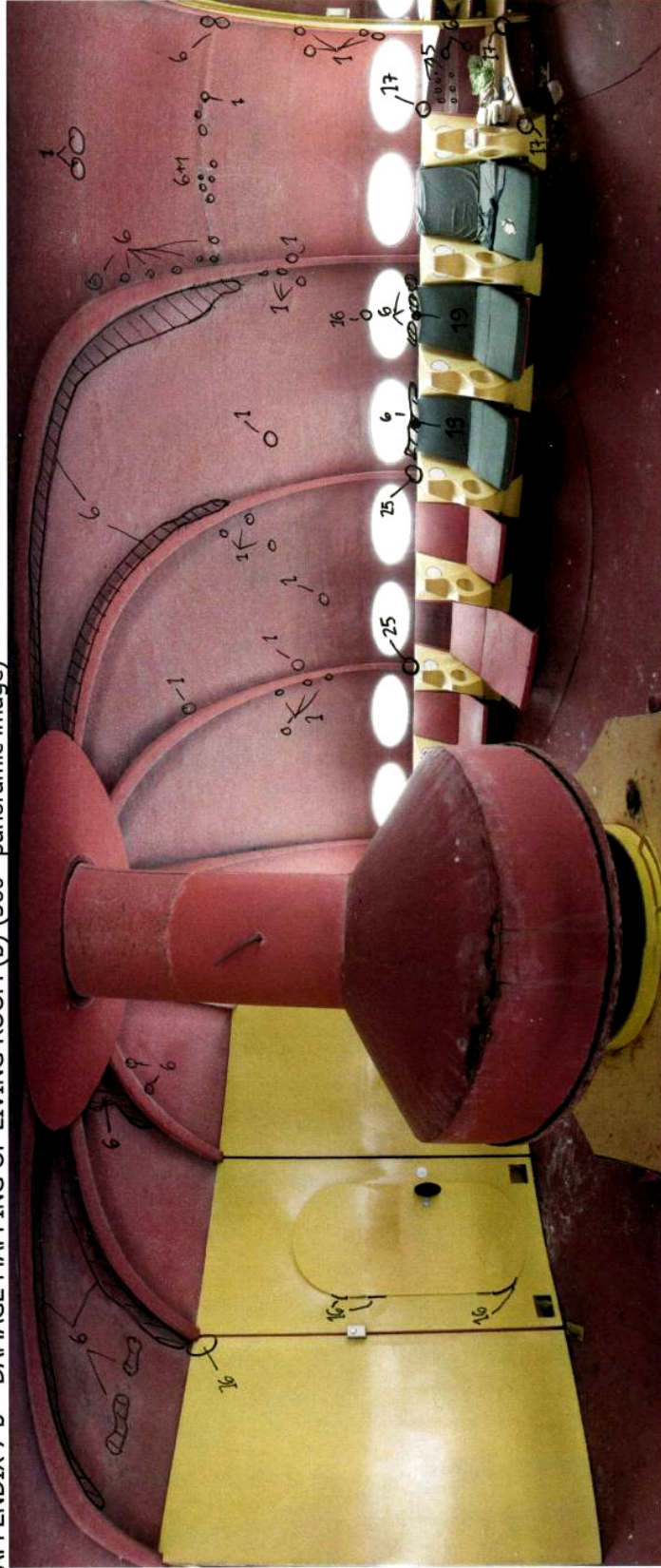
APPENDIX 7 b – DAMAGE MAPPING OF LIVING ROOM (b) (360° panoramic image)
