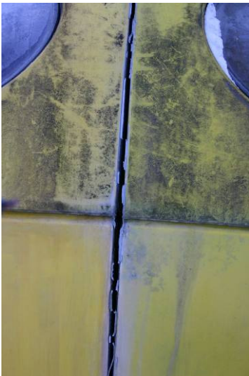
Figure 88. Many gaskets are cracked.
