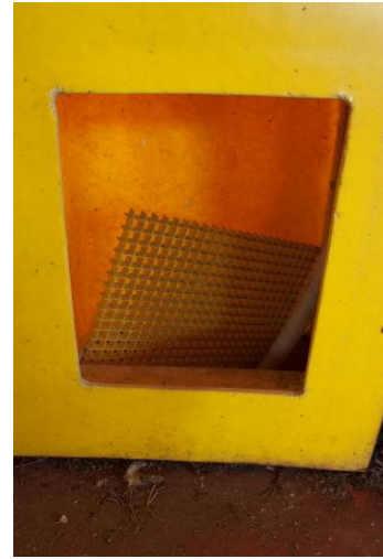
Figure 121. Loose grating on the ventilation hole.
