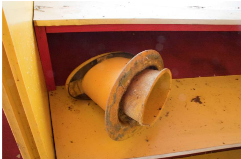
Figure 89. Protective cap of the air outlet has fallen down from the roof.
