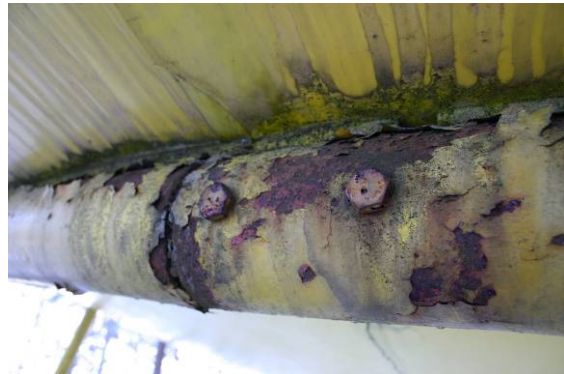
Figure 91. Corroded steel ring.
