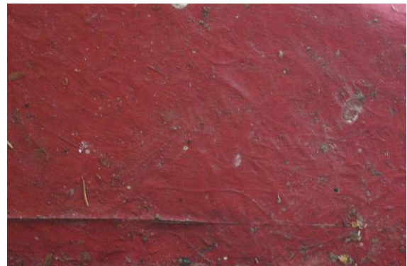
Figure 39. Uneven interior surface.
