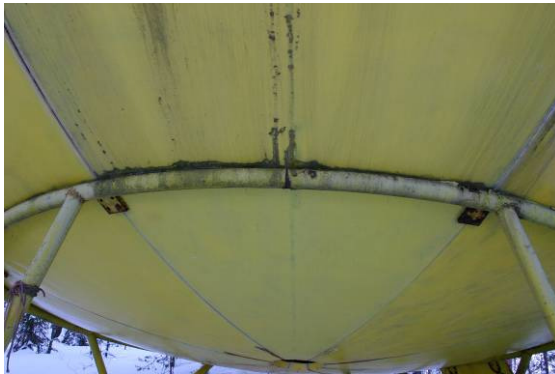
Figure 90. Steel ring is dirty and paint layer is coming off.
