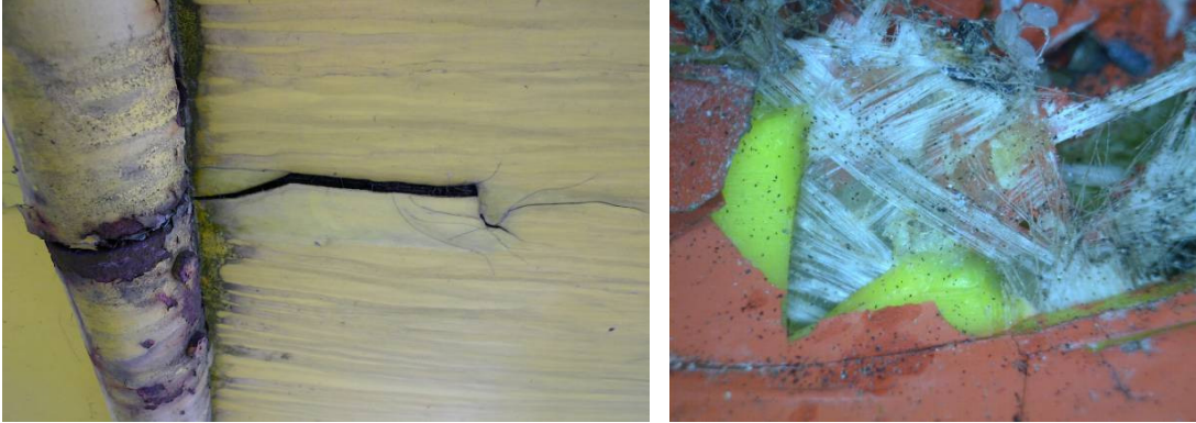
Figure 96. (left) Crack on the gel-coat on the bottom of the house.
