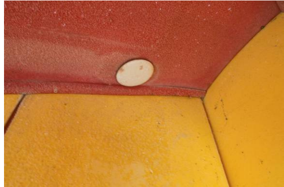
Figure 64. Air outlet in the ceiling.
