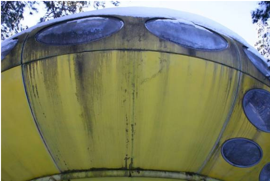
Figure 92. Dirt is concentrated mainly around the windows.
