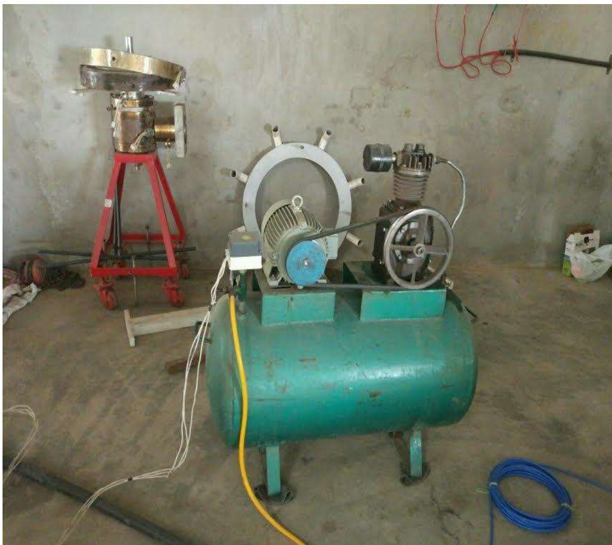
Figure 10. Air compressor at Seti Plastics (Nishan Devkota, 2017)
