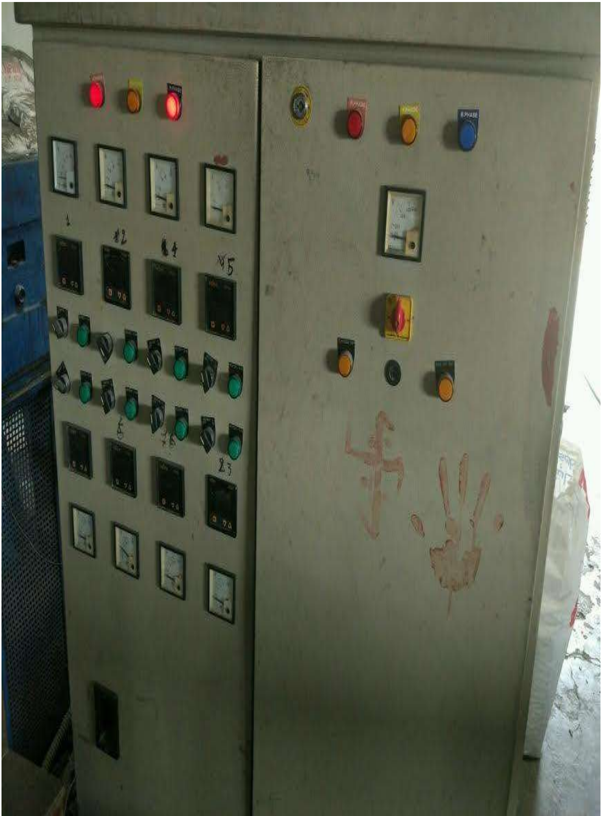
Figure 12. On-off temperature control II at Seti Plastics (Nishan Devkota, 2017)
