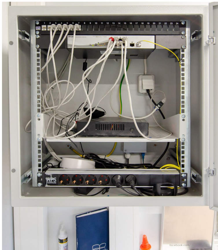
Figure 10: Case farm 4 network cabinet
