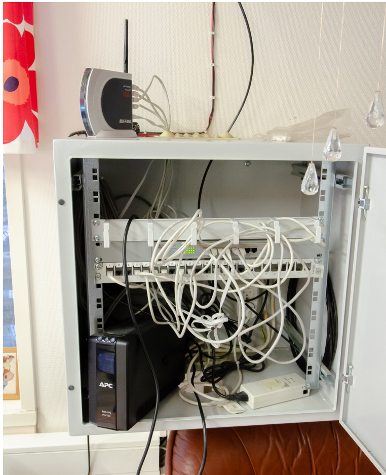
Figure 8. Case farm 3 network cabinet
