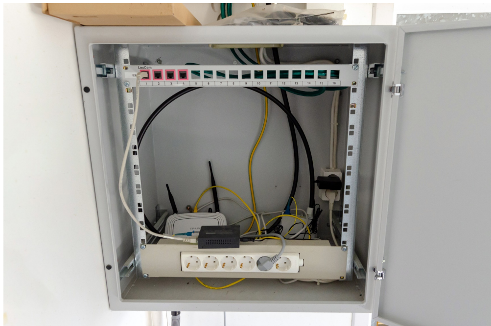
Figure 4. Case farm 1 network cabinet
