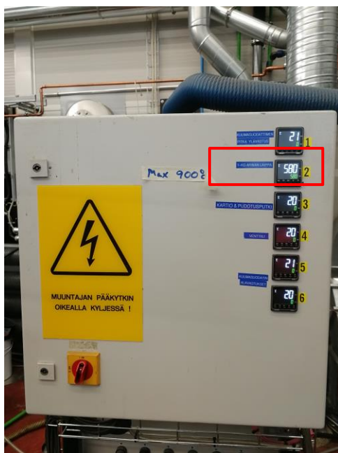
Image 7. Temperature control panel.
