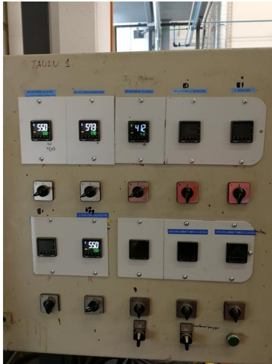
Image 8. Temperature control panel.
