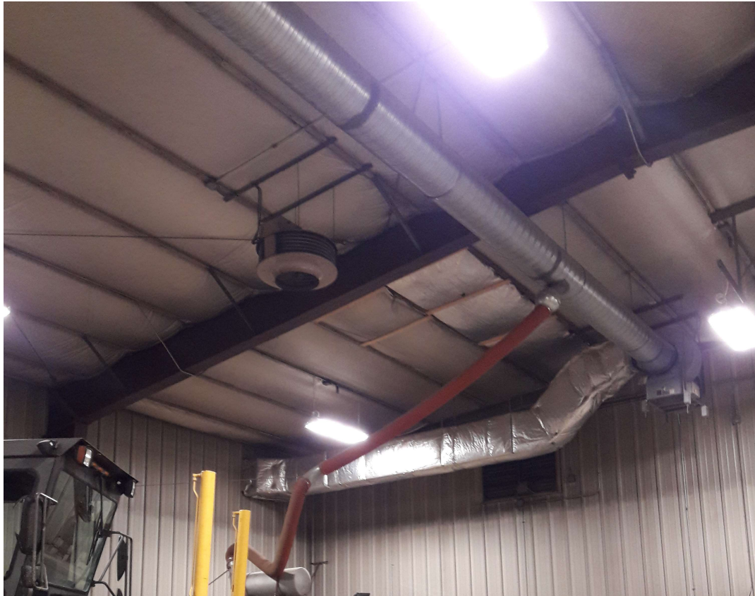
Picture 5. Hot air blowers in the Public Works Garage.
