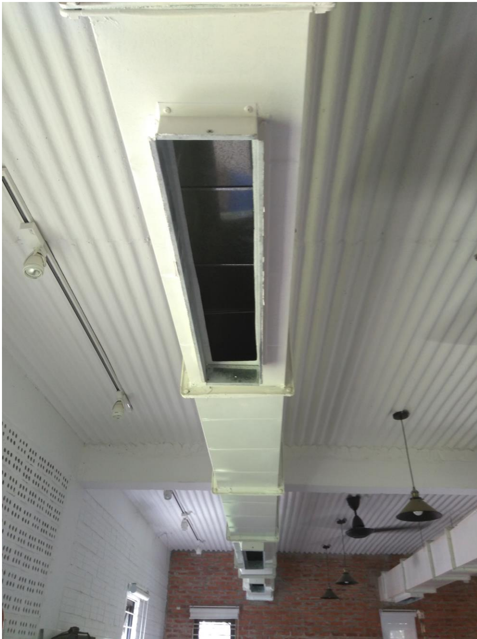
Figure 38. Ventilation pipeline connected to the central fan inside the Alpes building
