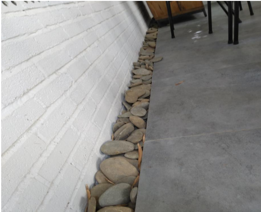
Figure 19. Wall water drainage inside the Alpes building
