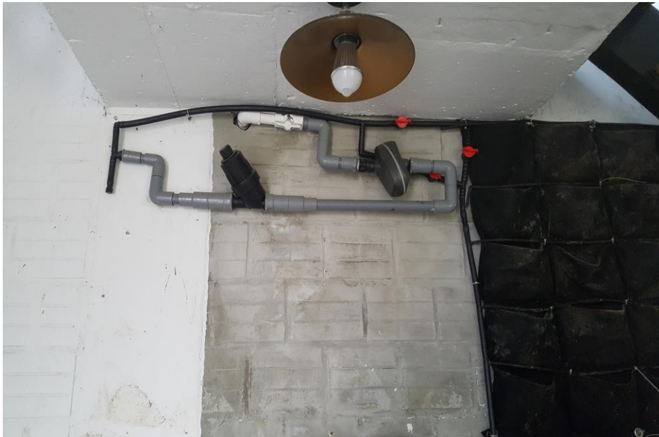
Figure 50. Automatic irrigation system of the Alpes building
