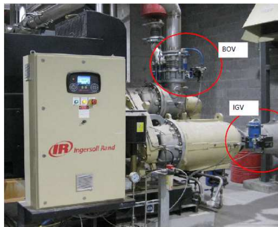
Figure 9. Both IGV and BOV seen on the compressor.
