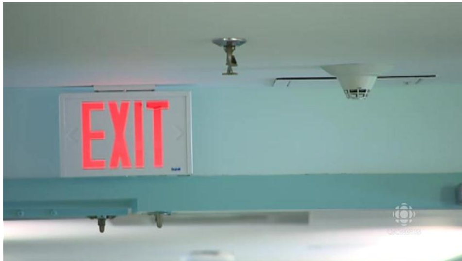
Figure 17. Smoke detector (right), sprinkler (middle) (CBC, 2014)
