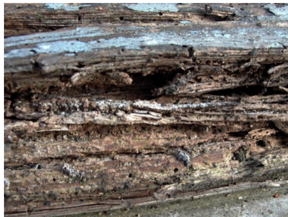
Figure 6. Rotten wood (rosebud10, 2006)
