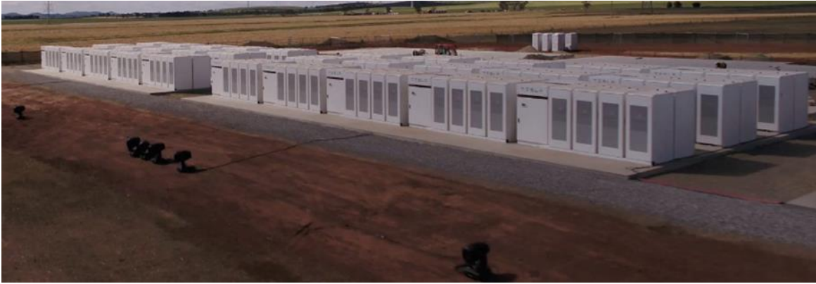
FIGURE 9. Tesla 100MW/129 MWh Powerpack battery (Lambert 2018).
