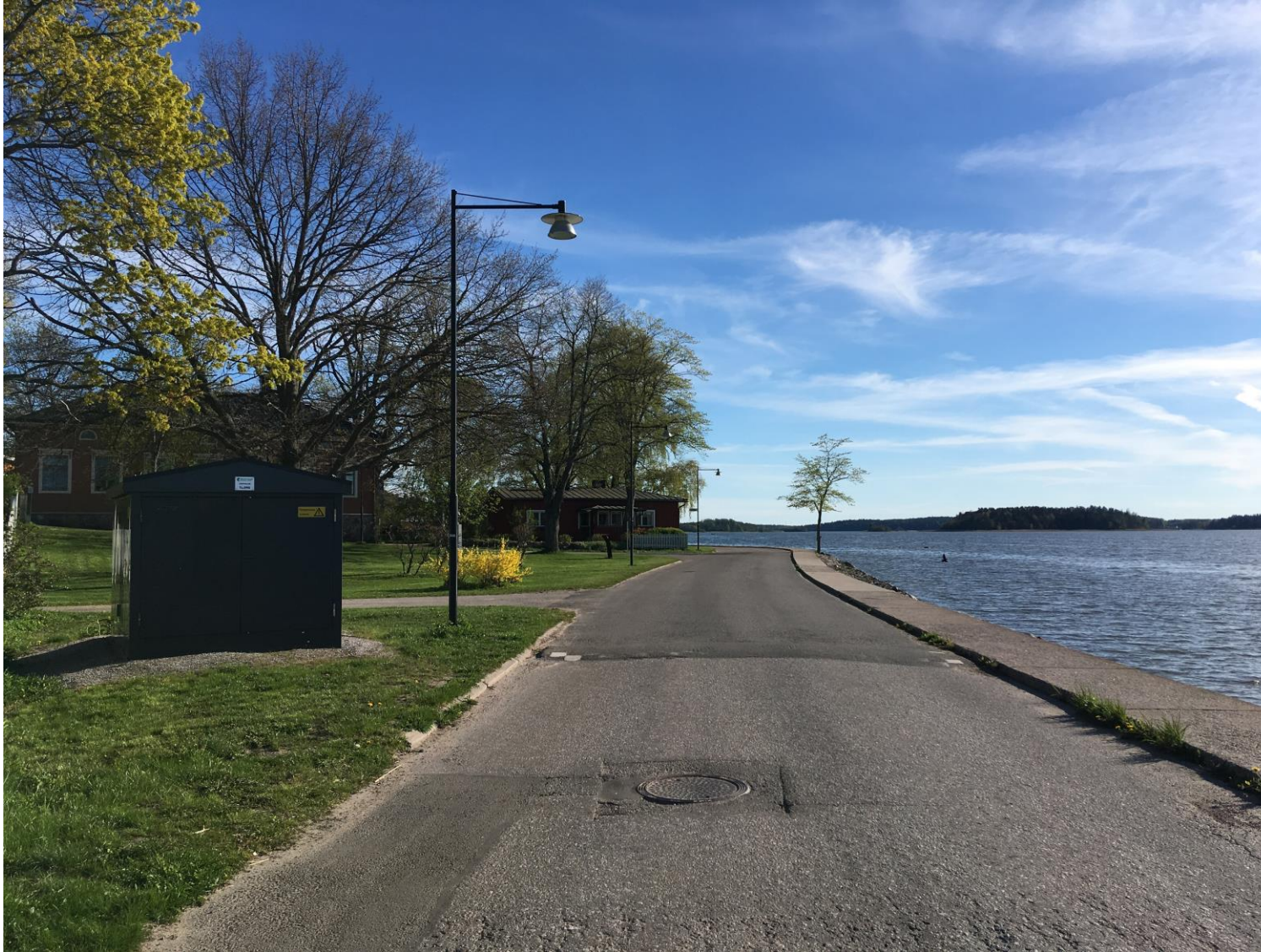
Appendix 25: Power distribution box near Västvallen Road. Photo by: © Jack Räisänen. Photo taken on May 15, 2019.
