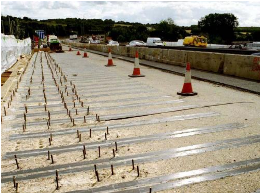
Figure 6.5 Example of strengthening made above the structure (Teke brochure “Structure strengthening with composites”)
