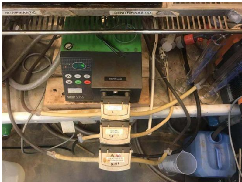
Figure 19. The pump of Influent, ANOX and return sludge
